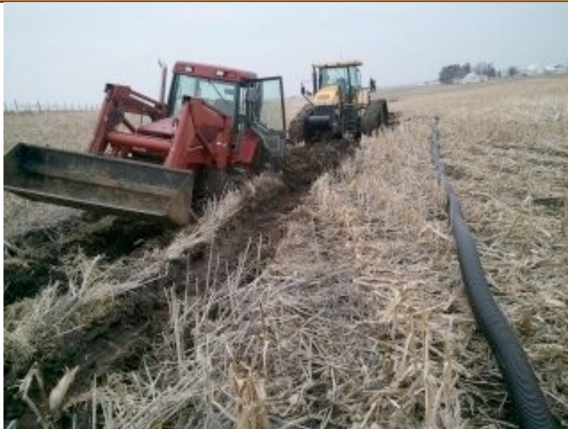
Little wet here, not now with the tile
